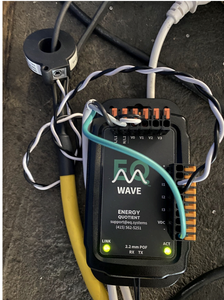
Figure 1: EQ Wave v1.1 install at JIFX 26-3, McMillan hangar. The Intellimeter CT (upper left) is clamped around the line conductor exposed by the measurement line splitter. The L/N terminals power the Wave (~2.5 W); L and N are jumpered to V1 and V0 for voltage sensing. Optical-fiber uplink active (both indicator LEDs green).
